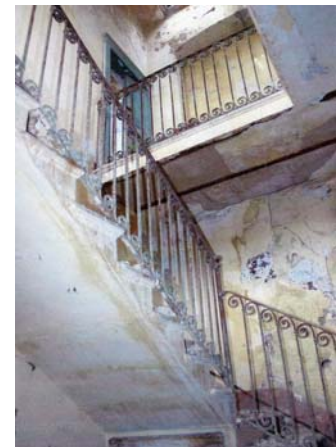
The door at the top of the stairs was Col Davis' office
